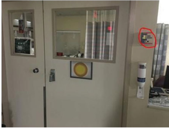
Fig. 5 Room pressurization monitor outside door (circled red)
